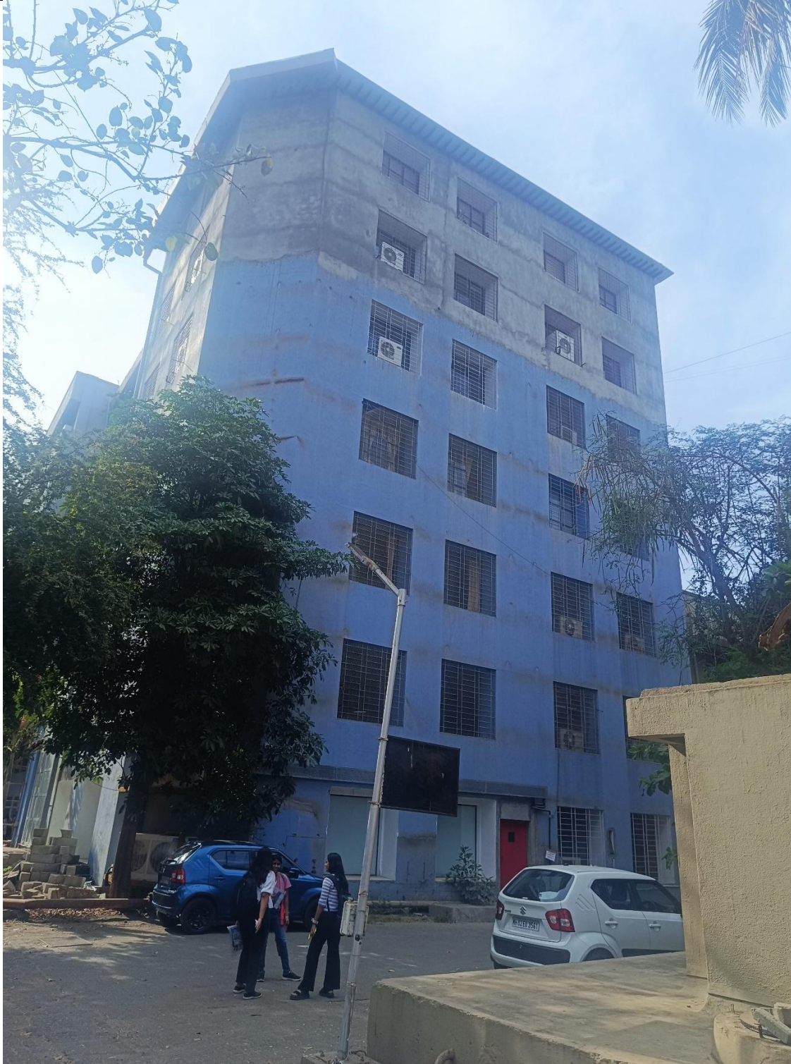
Photograph showing EAST wing where we have recently expanded existing G=4 to G+6 within 4 months including interiors
